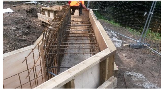
The foundations, abutments and wing walls were formed with shutters and reinforced concrete.
