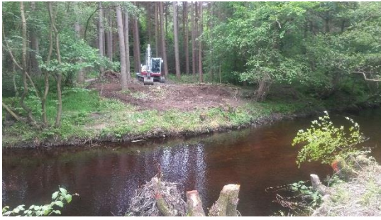
Trees were removed from the riverbank, and excavations were made for the abutments.
