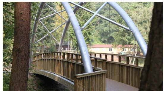
Timber was used for the deck and handrails. The bridge was then surfaced with tarmac and a resin top.
