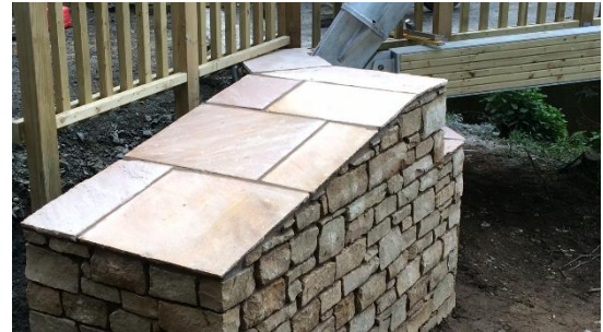
All exposed concrete on the abutments and wing walls was clad in sandstone.
