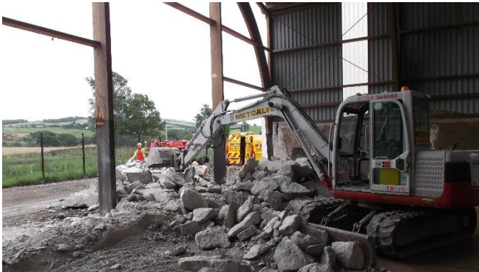
The cladding was removed by hand using a MEWP, before the end of the retaining wall was carefully demolished ready for the extension.
