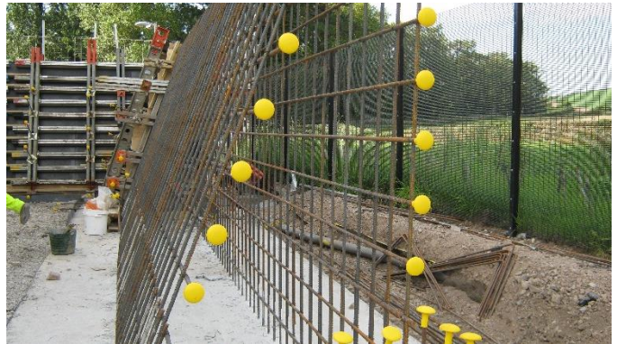
The retaining wall was extended using cast in-situ concrete. The wall was over 3m high, 1m wide at the bottom and 300mm at the top.
