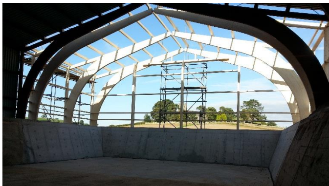
The new walls and polished concrete floor, with the Glulam beams visible.
