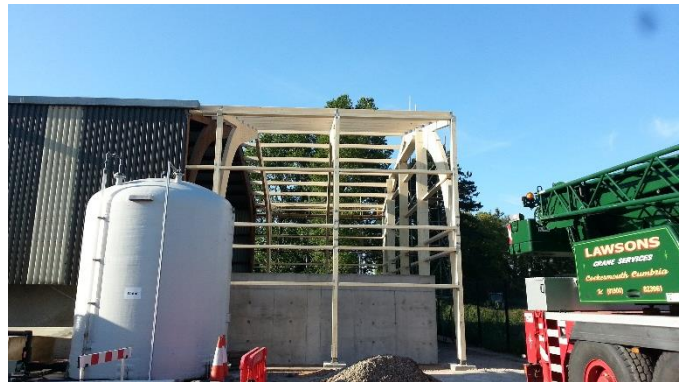
A side view of the Glulam work. Cladding was finally added to match the existing structure.
