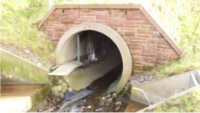
The existing Otter Ledge had been vandalised and set on fire. The first job was to remove and dispose of it.
