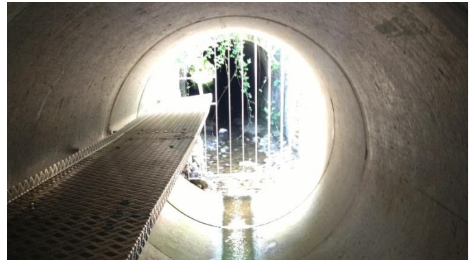
The finished Otter Ledge and downstream trash screen. The screen was constructed in two parts so we could carry it down the pipe.
