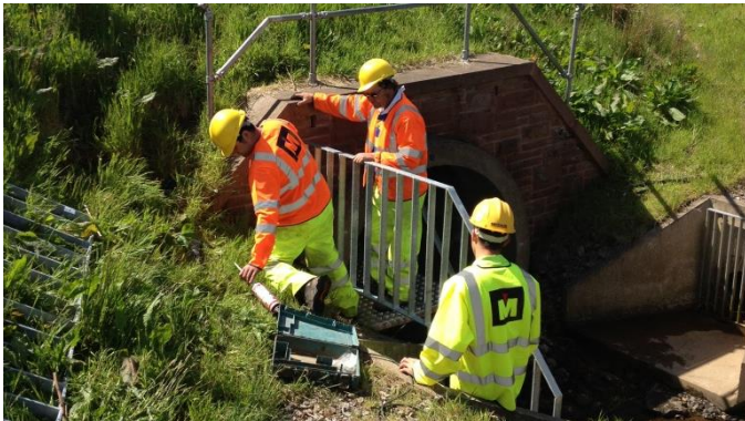
The trash screen at the upstream end was difficult to design and install because of its complicated shape and the difficult site access.
