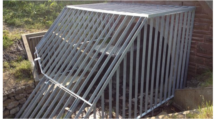
The finished screen should stop any damage to the ledge, caused by either debris flowing downstream or vandalism.
