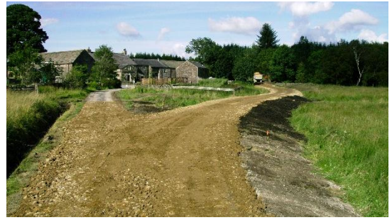
The finished bypass road allowed for the stone to be hauled to the new car park and footpaths.
