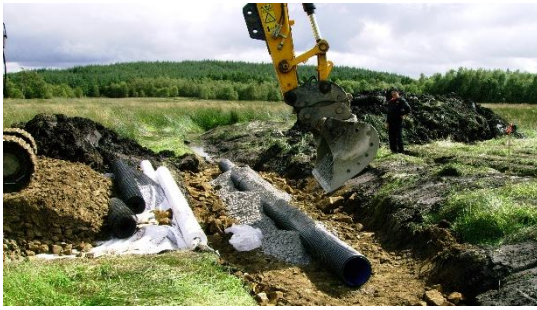
The bypass road was constructed over peat. It incorporated geogrid, geotextile and drainage.
