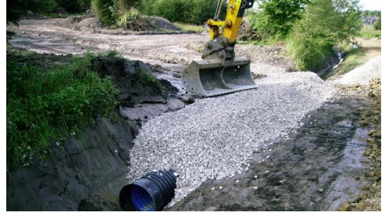
The car park was stripped and drainage installed including culvert crossings. Stone was used to surface it.
