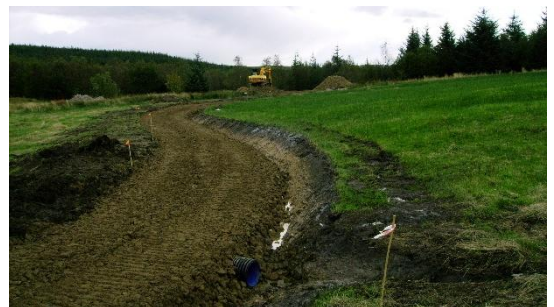
Foot and beginners cycle paths were also created using stone from the quarry. This area required much drainage.
