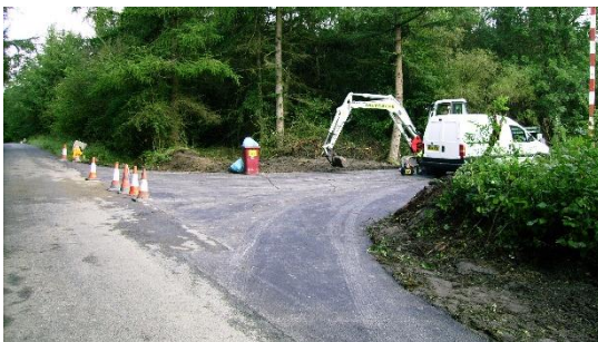
The main entrance to the forest was widened and resurfaced ready for use by the public.
