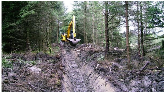
A cut off ditch was constructed above the top edge of the car park. On this site water was a constant problem.
