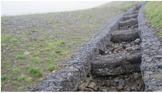
The original cascade had been formed using gabion baskets which had failed due to high water volumes.
