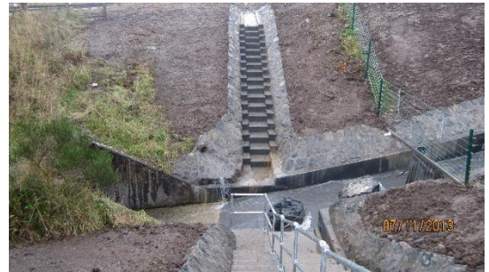
The two finished cascades allowed water to drain into the main channel. Handrails were installed on the steps.
