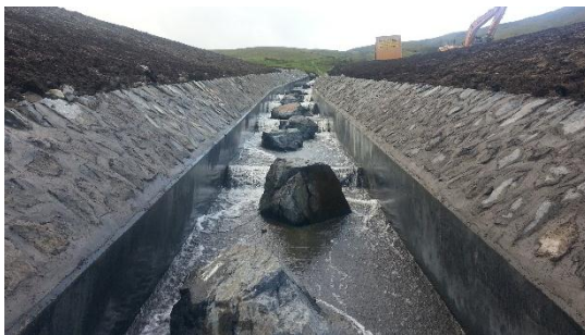
The tops of the cascades were stone pitched to retain the existing ground and provide additional capacity.
