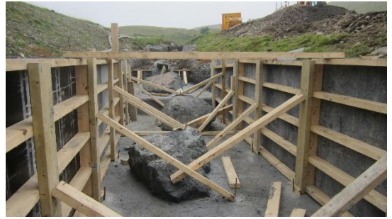
The main cascade was constructed using shuttered concrete with the water over pumped around the site.
