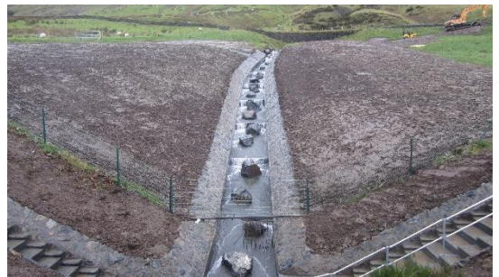
The site was then re-graded and reinstated with topsoil back to original levels.
