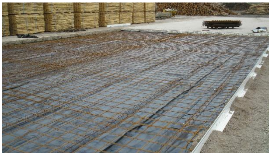
MPH's concreting gang formed the slab in 9m wide strips, including reinforcement and construction joints.
