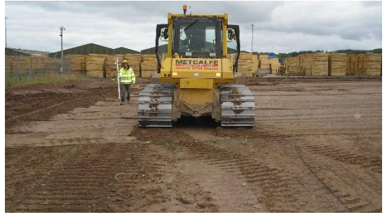
The existing subsoil was trimmed to a good level ready for the soil stabilisation contractor.
