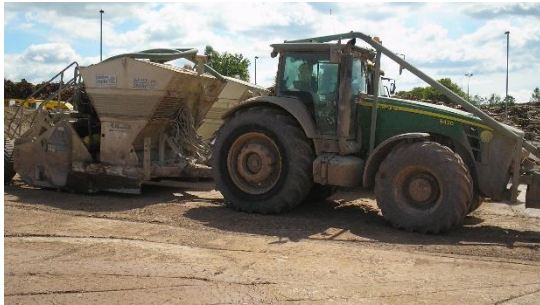
MPH hired a soil stabilisation specialist to improve the subgrade. This reduced spoil and saved on capping stone.
