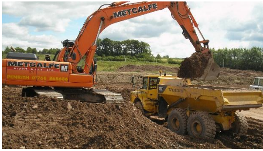
Bulk earthworks were done to cut and fill the area to suitable levels.
