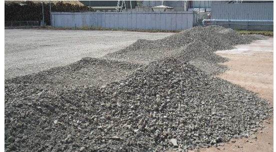
A thinner layer of sub-base was used to trim to the finished formation level.
