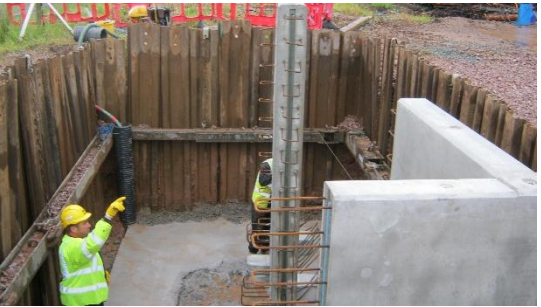
The solids separator was mainly precast, with the corners cast on site. The excavation was supported with shoring.
