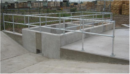
The finished tank. Handrails were installed to protect operatives when inspecting or cleaning the tank.
