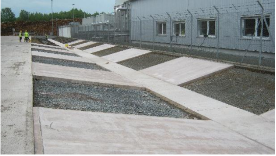
The channel was formed in a checkerboard pattern with mesh in the bottom and dowelled joints along the edges.
