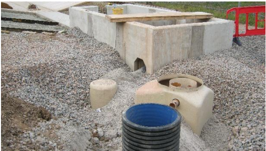
The interceptor was installed afterwards. The whole area was concreted to allow access.
