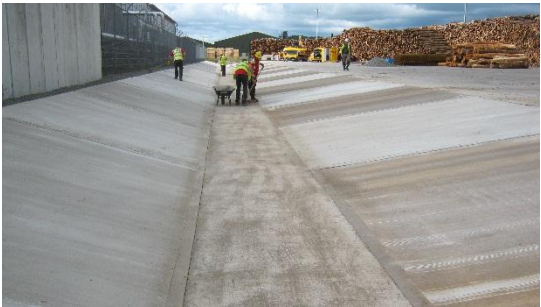
The finished channel was designed to fall towards a new 'solids separator' and traditional oil interceptor tank.
