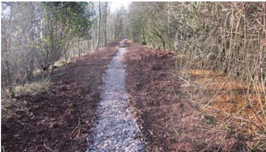
Another finished filter drain. This was one of a number of field and top batter drains repaired or replaced
