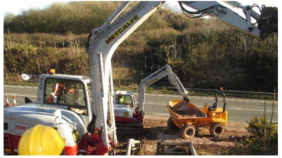
Drains at the top of batters, in surrounding fields and other small drains were repaired where necessary.
