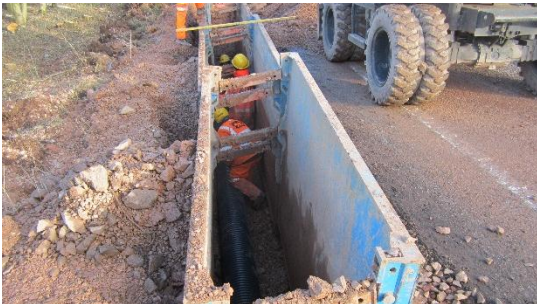
Working in made-up ground meant trench support was needed for a lot of the excavations.
