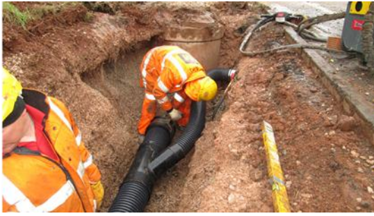
The repairs were to carrier and filter drains, in small sections as well as long runs between manholes.
