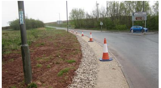
A finished section of filter drain. Sub-base was used to trim the edge next to the carriageway.
