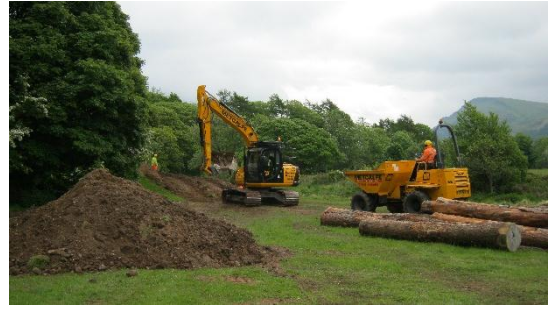
Rock armour (rip rap) stone and logs were delivered to site and taken down in dumpers.
