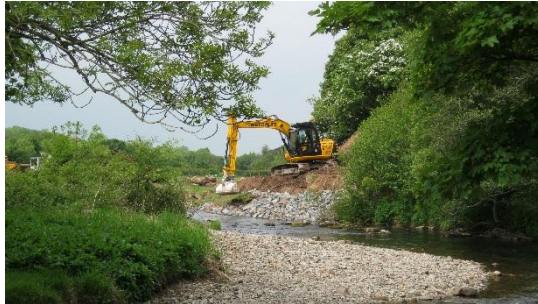
The rock armour was placed at the toe of the higher banking.
