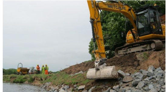
Topsoil was used above the rock armour and the logs to re-profile the embankment.
