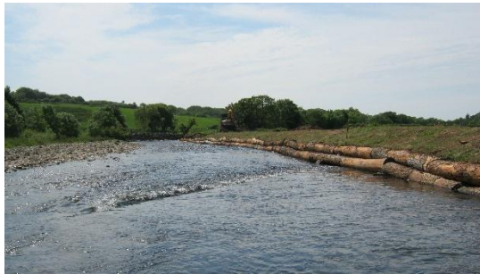
The logs were pre-drilled and lifted into place, then secured with steel pins.
