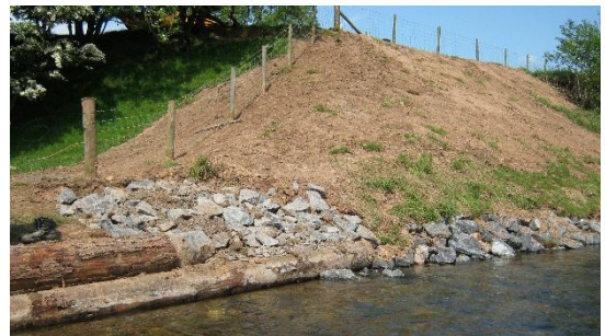
The logs were used on the shallow section and blended into the rock armour section.
