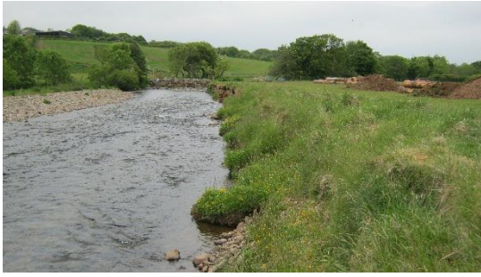
The existing riverbank was eroding during floods, destroying the land on the outside of the bend.
