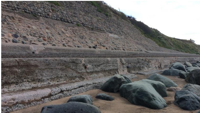
The existing sea wall was beginning to show signs of wear, and required a new concrete face.
