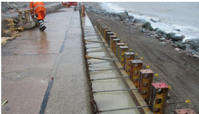
The top lift was attached to the bottom and the existing wall.
