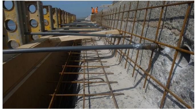
The first lift of concrete was fastened to the foundation and the existing wall. Steel mesh and L-bars ensured a permanent hold.
